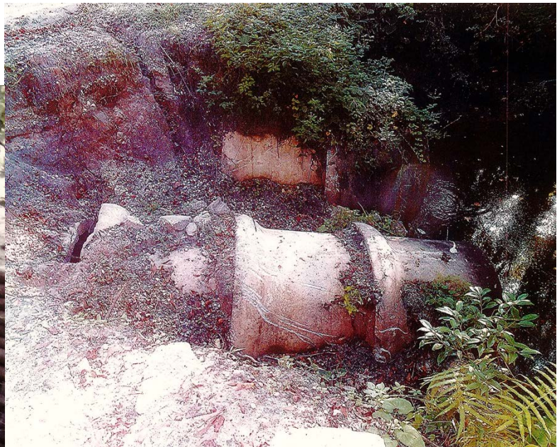
Before the Repairs
